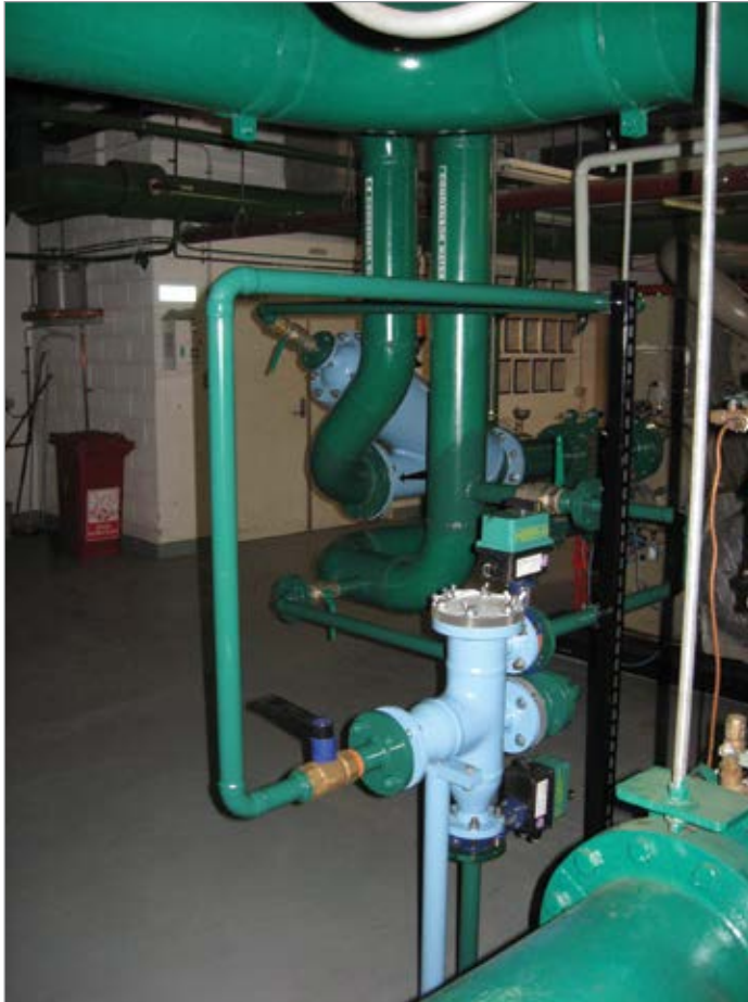
Figure 5: The sponge ball ATCS installed in Case 1
