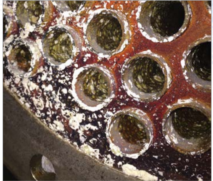
Figure 1: Severe fouling of water cooled condenser tubes.
