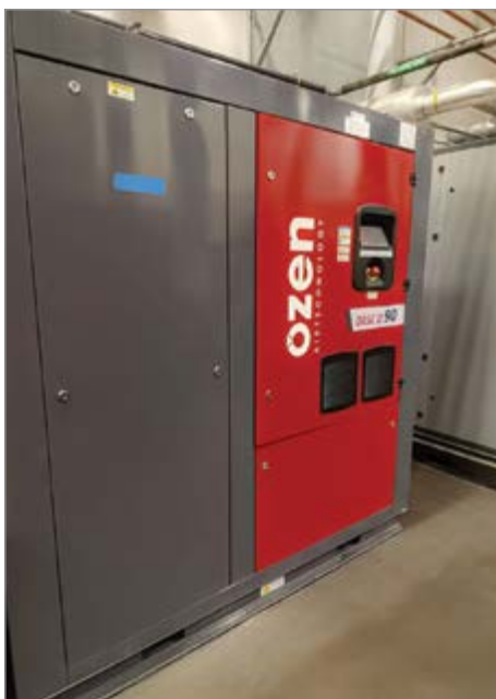
A nitrogen generator is fed by this variable frequency drive air compressor
