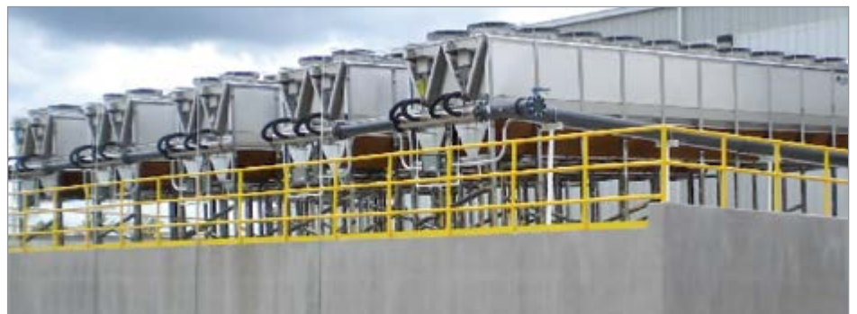
A self-draining adiabatic cooling system
