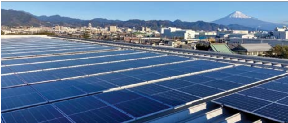
Solar panels installed at the Shimizu Works (Shizuoka City, Shizuoka Prefecture, Japan)
