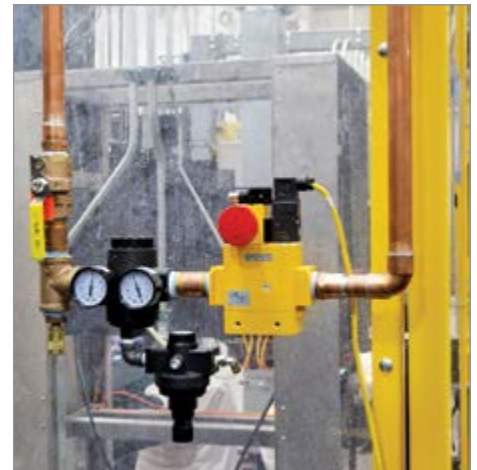
A flow controller on a compressed air system
