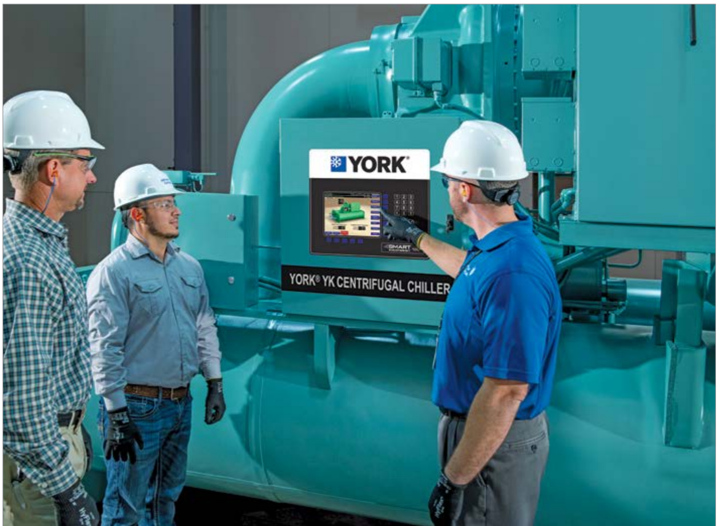
Most modern high-efficiency chillers use variable speed drives to vary the chiller's capacity.
